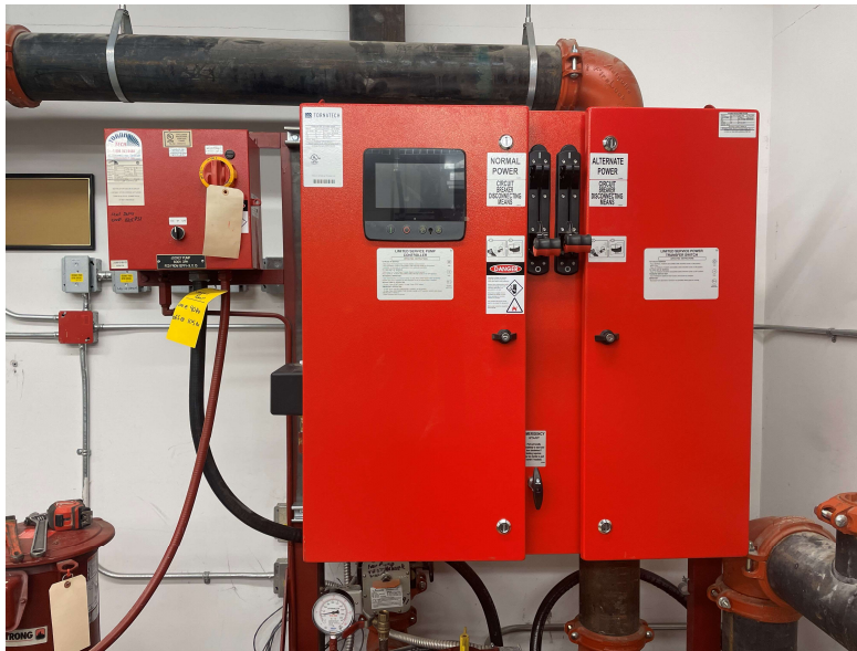
New Fire Pump / Panel System
