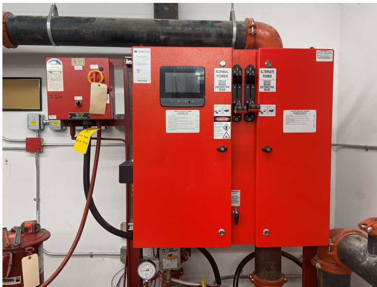
New Fire Pump / Panel System
